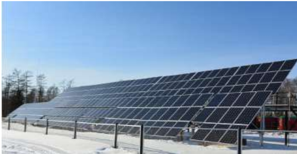
Figure 4.22 60 kW autonomous solar plant in Batamai
